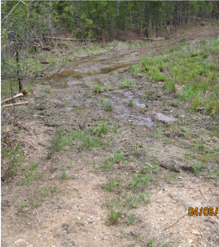
FIGURE 5.5. AREA OF SEEPAGE NEAR TOE OF DAM.
