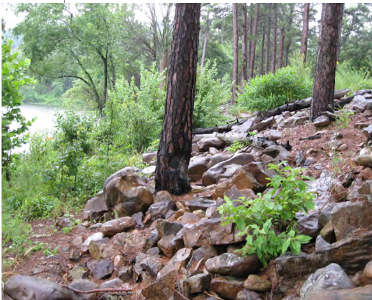
FIGURE 7.3. TREES AND WOODY BRUSH GROWING ON THE DAM.
