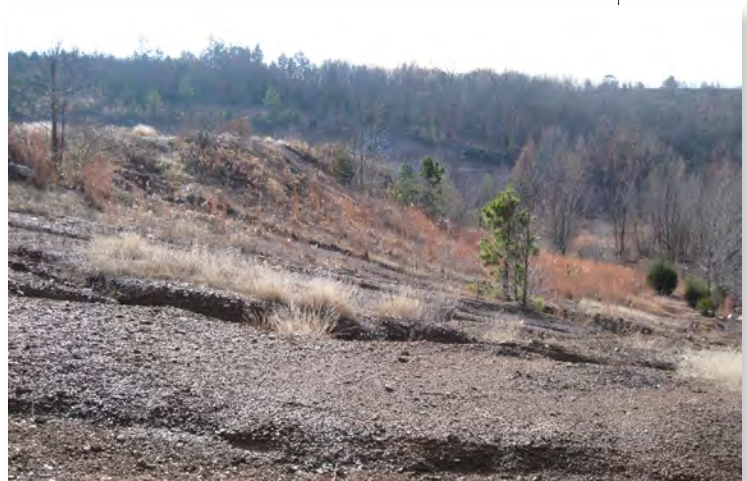
FIGURE 7.1. EROSION OF EMBANKMENT WITH POOR COVER
