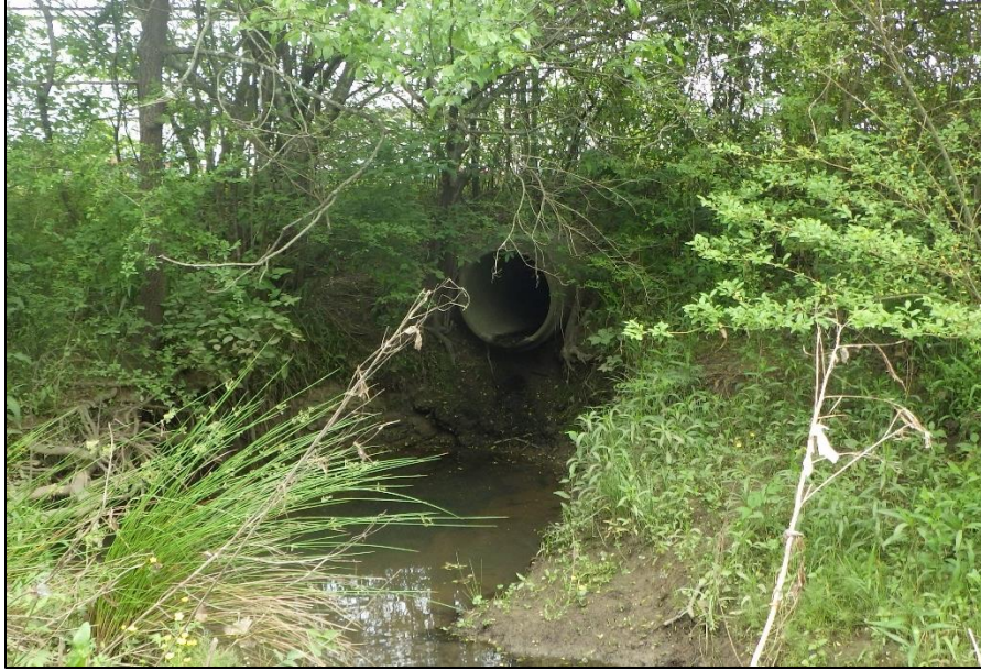
Figure 3.2.3. Typical Storm Water Outfall from an Urban Area in Little Creek.
